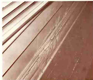
Figure 3 Cracked and warped baseboard decayed by Poria .
