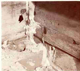
Figure 2 Rhizomorph (arrowed) emerging through masonry from earth-filled porch.
