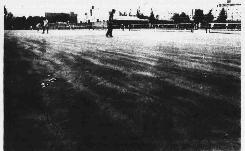
Six of the tennis courts beside Carmichael are falling prey to the shifting ground they were built upon, which was once a marsh. As the courts go under, large cracks are left in the surfaces.
