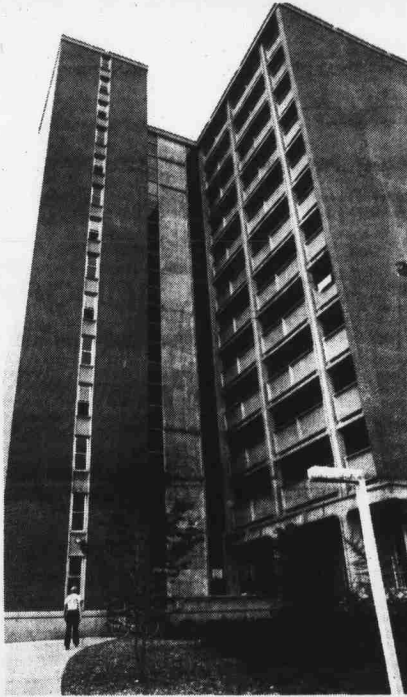
The Physical Plant was forced to remove 12 floors of brick veneer (gray area in center) from the Sullivan elevator tower when it was discovered that the brick was separating from the concrete underneath.
