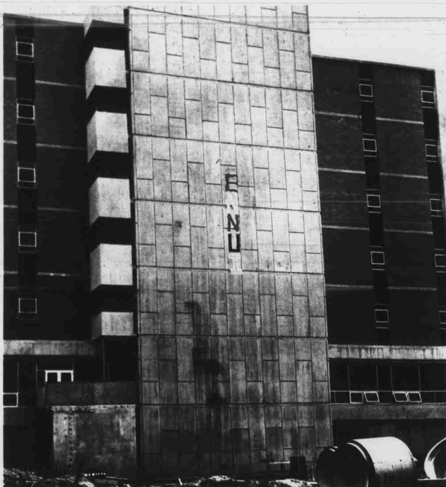
Ennu? According to the dictionary, ennu means a feeling of weariness or dissatisfaction. But how it got there no one knows. Operators on the construction site say it wasn't by means of the crane. It could have been done by ropes from the top of the building but Generals is locked at 5:00. (photo by Hankins)
