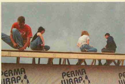
Brock Winstead, far left, shingling the roof. Courtesy of NCSU Habitat for Humanity
